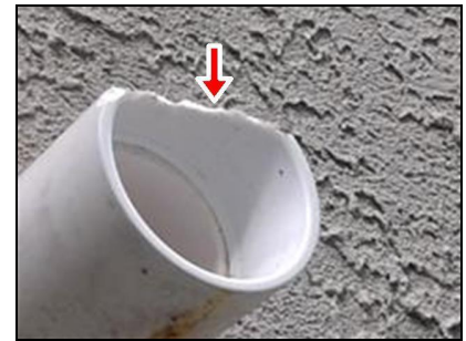
Water heater vent pipe
