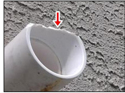
Water heater vent pipe
