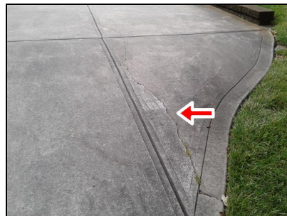
Typical cracking in driveway
