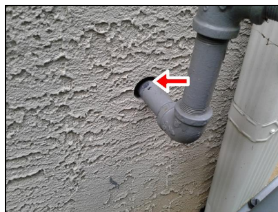
Gas line left side
