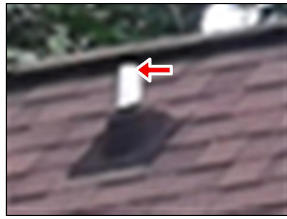
Plumbing vent pipe
