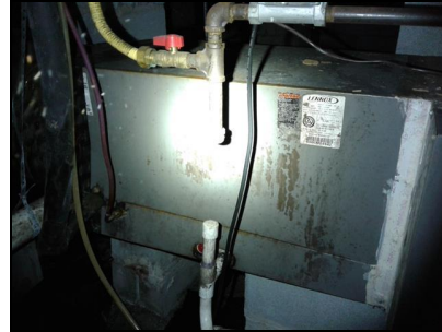
First floor indoor AC coil unit
