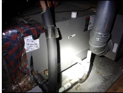
Second floor indoor AC coil unit
