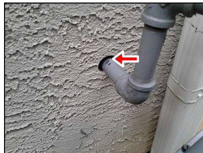
Gas line left side
