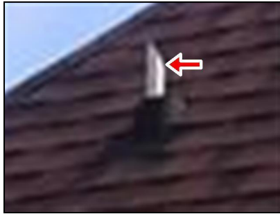
Plumbing vent pipe
