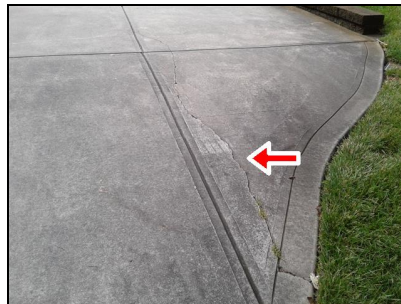
Typical cracking in driveway
