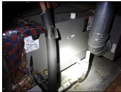
Second floor indoor AC coil unit
