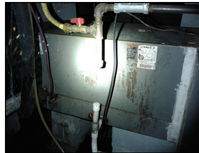
First floor indoor AC coil unit
