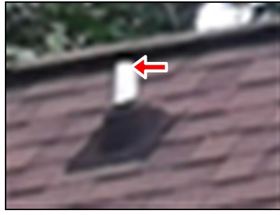
Plumbing vent pipe
