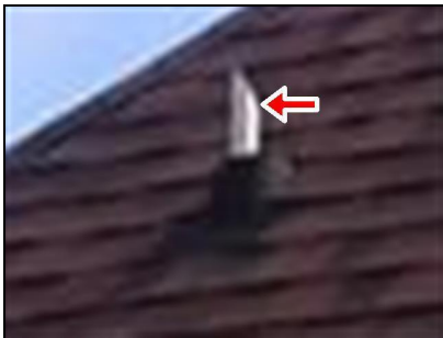
Plumbing vent pipe
