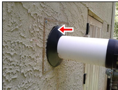
Tankless water heater vent
